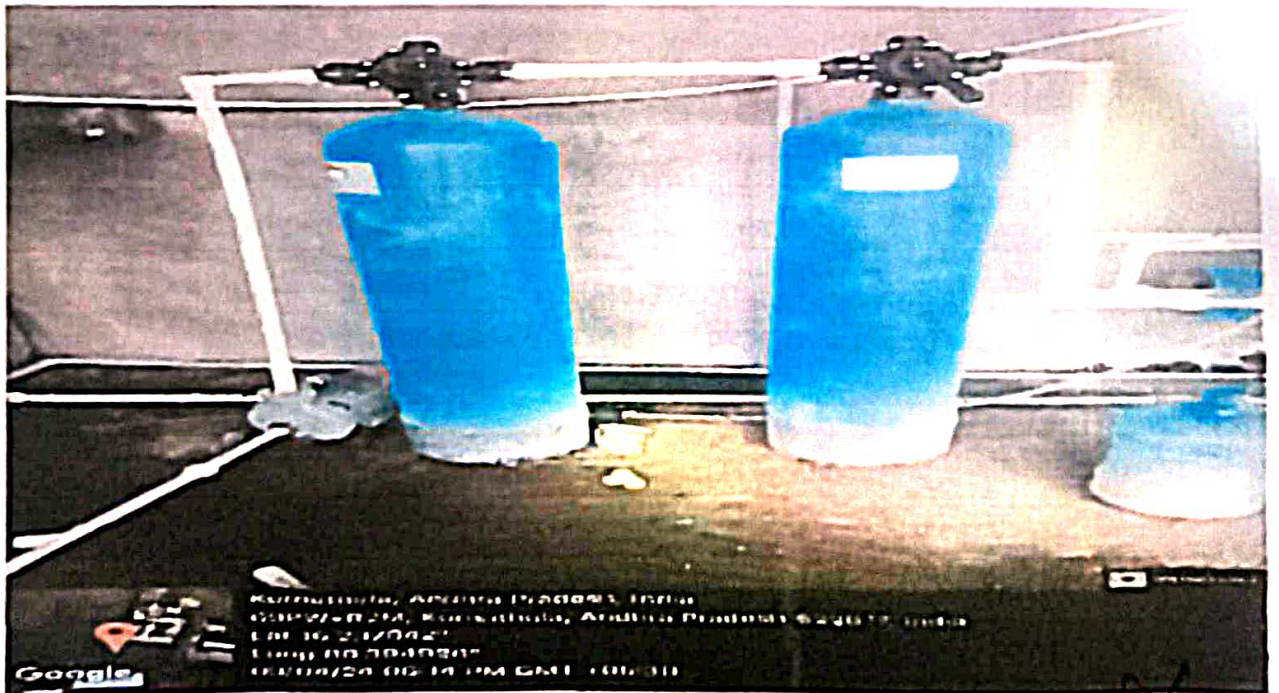
RO Water Plant
